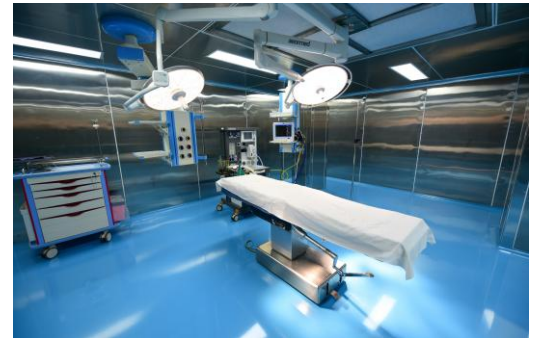
Modular Operation Theater Complex
